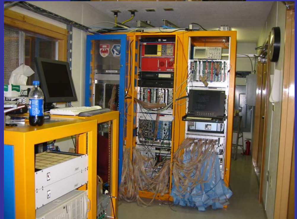
Electronics in Trailer
